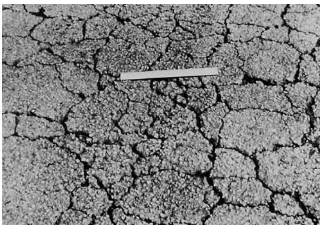
FIG. X1.3 High-Severity Alligator Cracking
