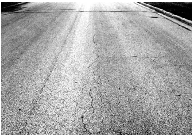
FIG. X1.1 Low-Severity Alligator Cracking
