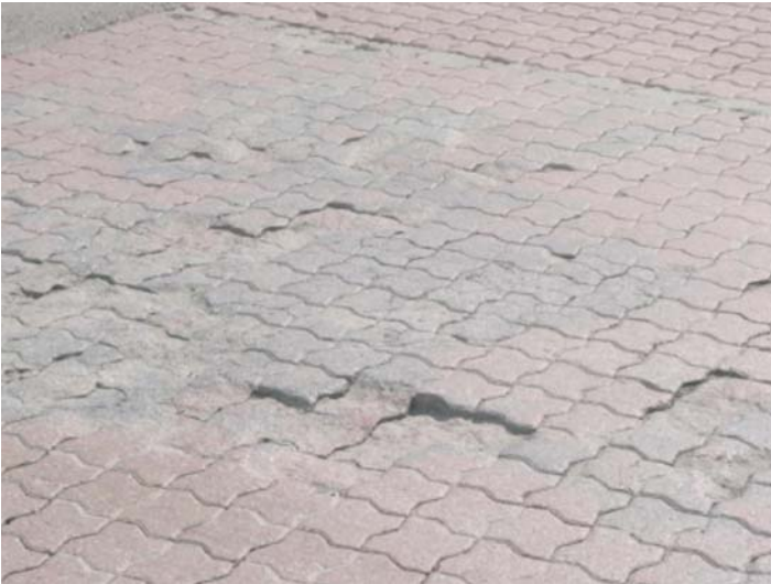
FIG. X1.3 High Severity Damaged Pavers
