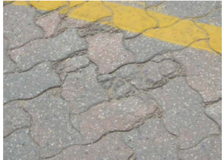
FIG. X1.2 Medium Severity Damaged Pavers
