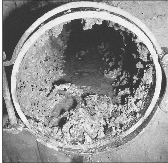
Figure 1-1 Pipe with tuberculation caused by corrosion
