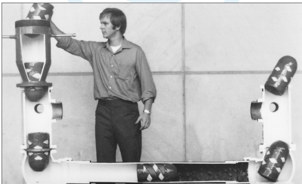
Figure 4-5 Pigs launched through a disassembled fire hydrant for a 6-in. (150-mm) or smaller line
