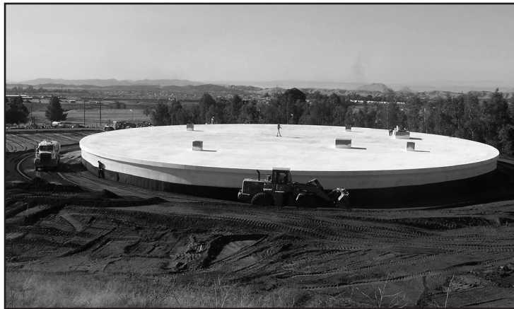
Figure I-3 Prestressed circular or cast-in-place rectangular reservoir (courtesy of Beaumont Cherry Valley Water District, J. Reichenberger, P.E., District Engineer)
