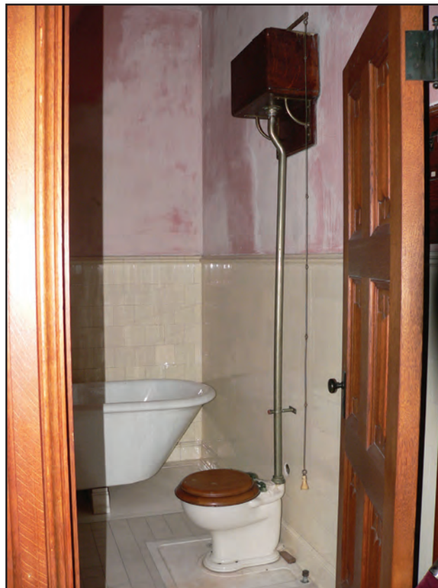
Figure 2-3 Old toilet technology
