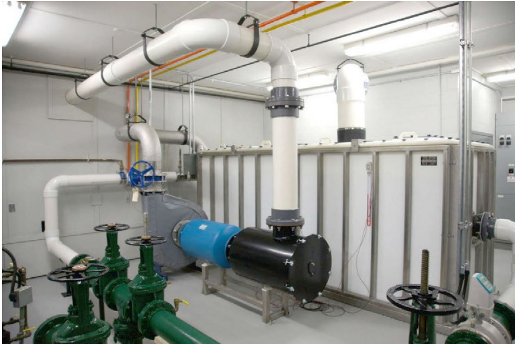
Figure 2-8 Multi-stage bubble system for the removal of carbon dioxide at 500 gpm (Searsport, Maine)
