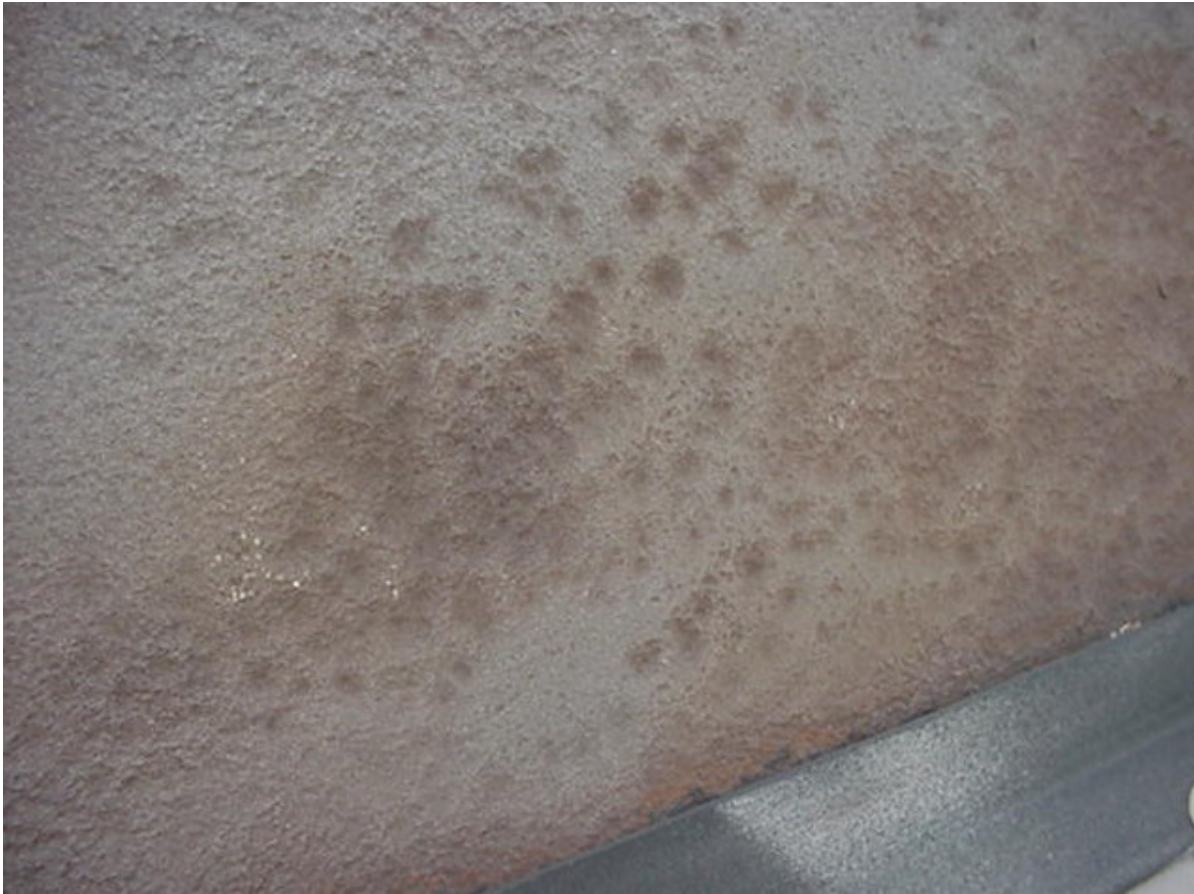
Figure 1 - Internal corrosion pitting on shell
