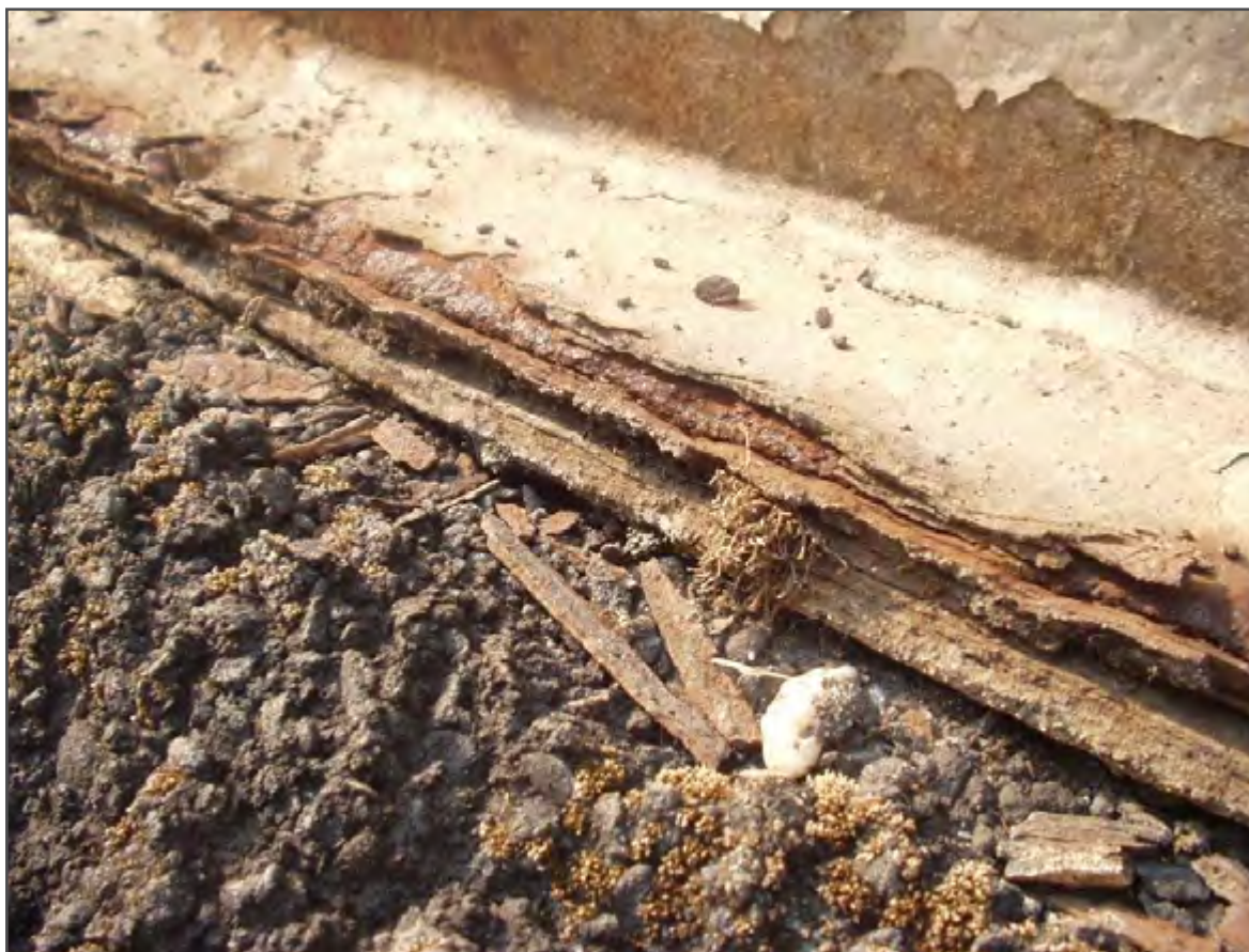
Figure 4-4 Under deposit corrosion tank annular projection
