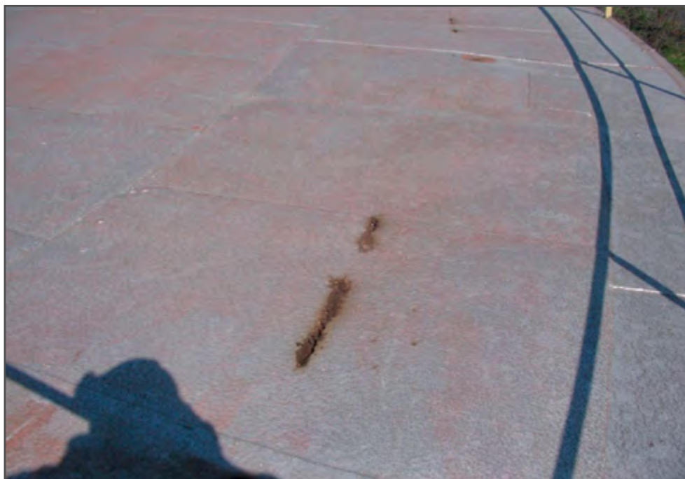
Figure 4-2 Crevice corrosion between roof supporting structures and roof plates in the vapour space of a tank that progressed to the top side of roof plates, even leading to holes
