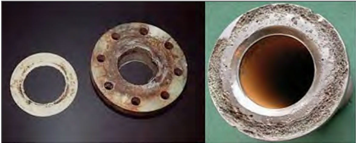
Figure 4-3 Corrosion at flange surfaces
