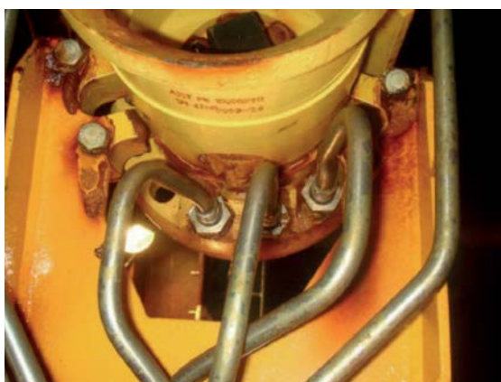
Figure 3 Umbilical connection head showing severe corrosion of the carbon steel components
