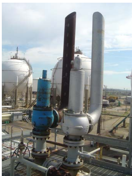
Photo 2 Safety valves showing local venting to atmosphere
