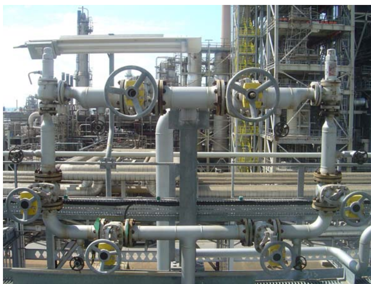
Photo 1 Safety valve isolation by using isolation valves along with a key operated interlock system
