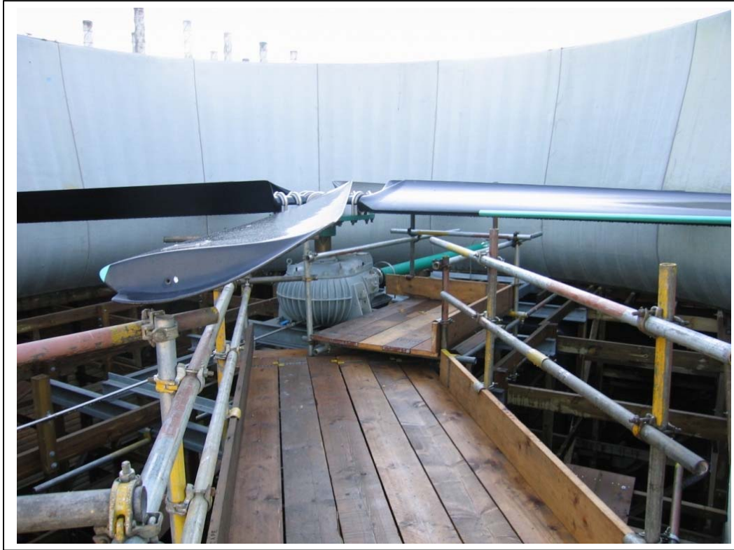
Figure 1 Typical industrial mechanical draught cooling tower fan
