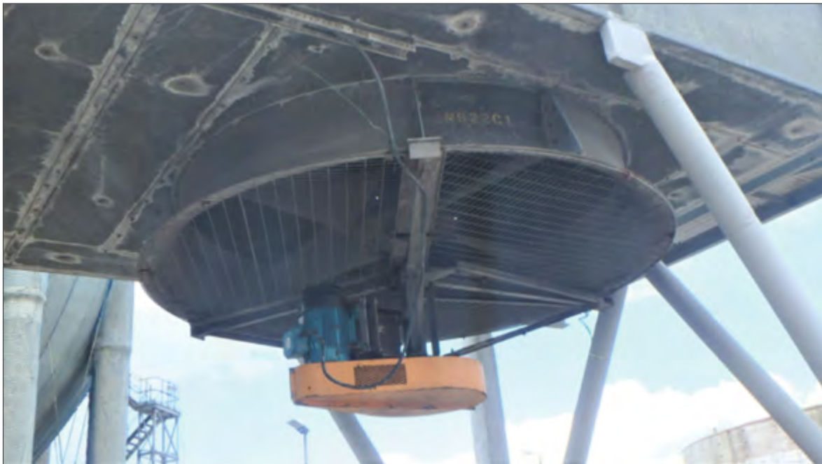
Figure 2 Typical fin fan unit
