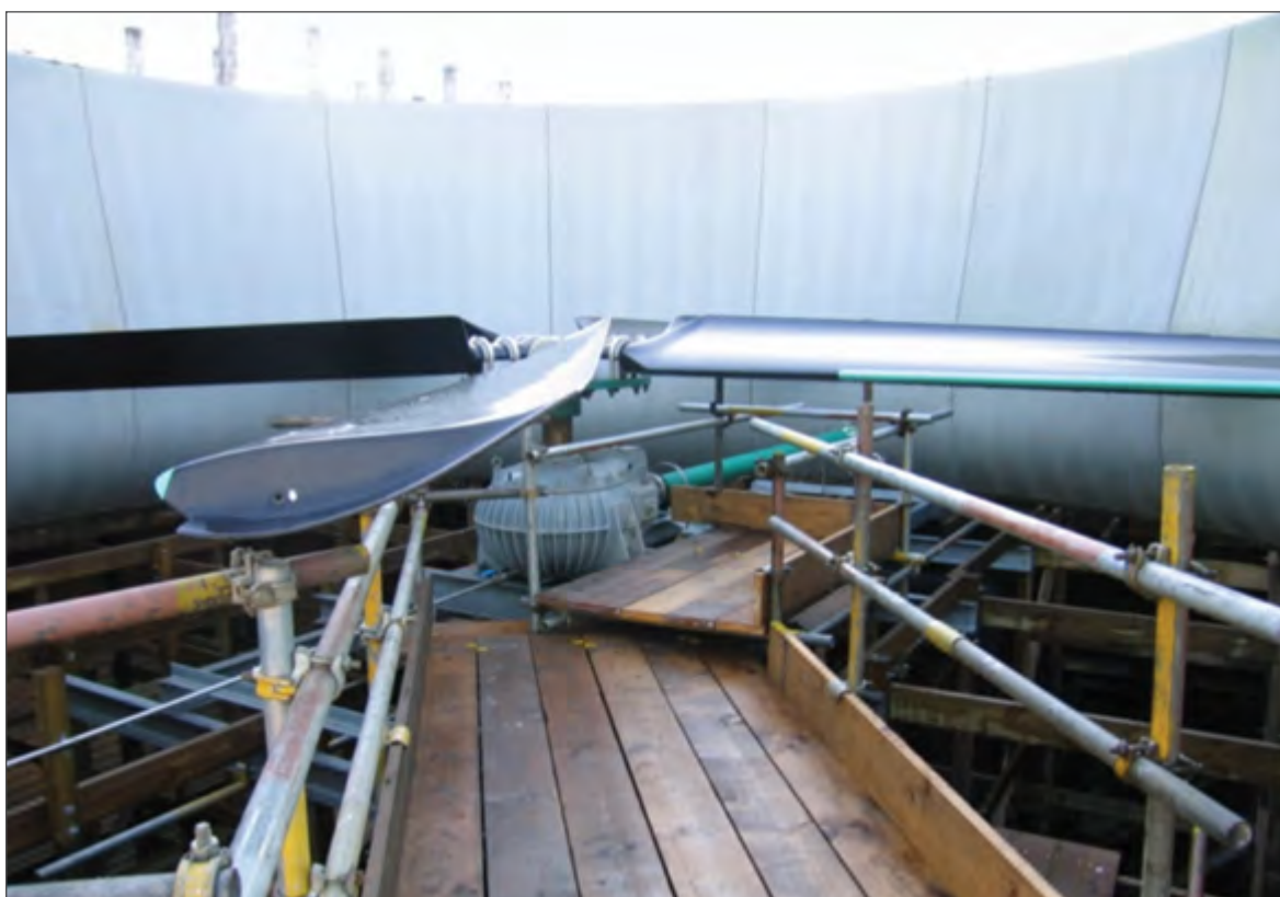
Figure 1 Typical industrial mechanical draught cooling tower fan
