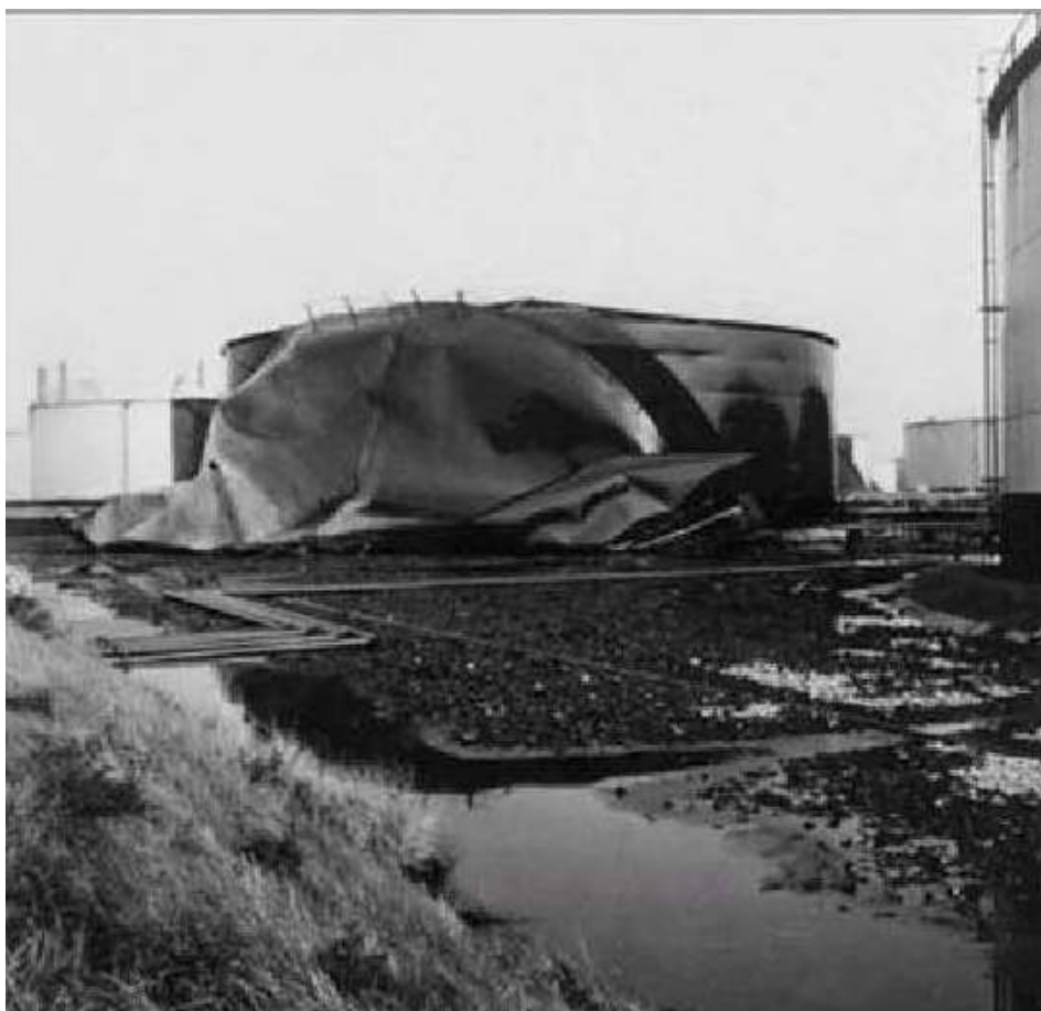
Figure 3 Tank collapse due to rapid temperature changes
