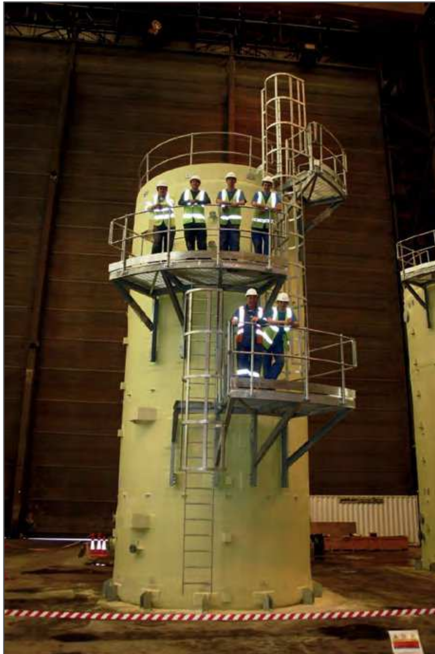
Figure 7: Tank showing access ladders, platforms and circular hand railing
