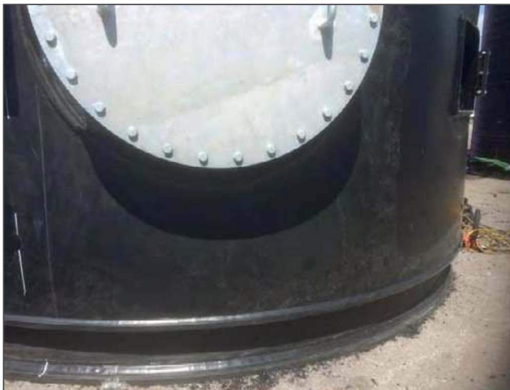
Figure 13: A thermoplastic tank insulated to 150mm above base level
