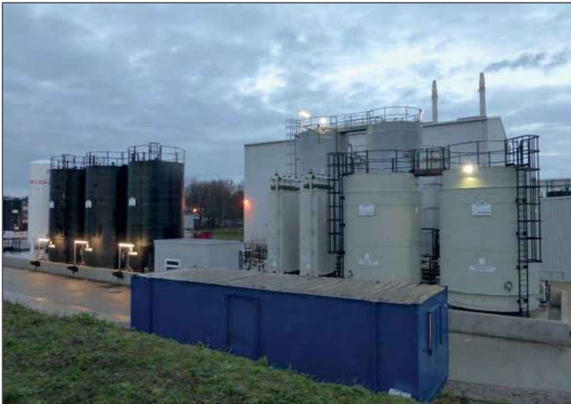
Figure 1: Installed polypropylene and high-density polyethylene tanks
