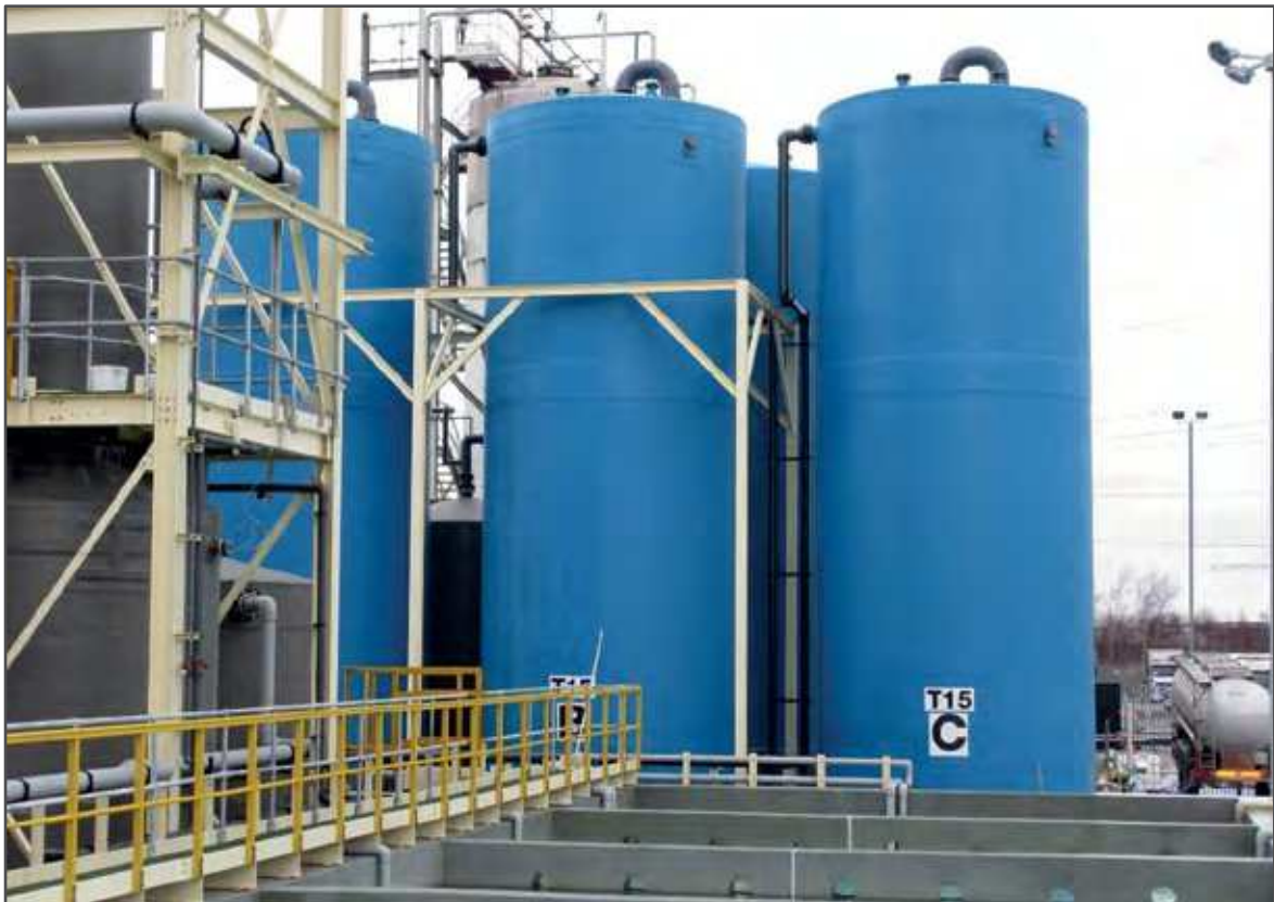
Figure 2: Installed GRP tanks
