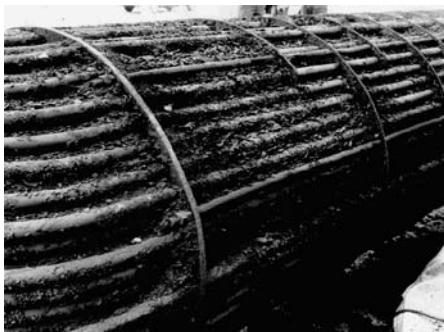
fouled heat exchanger
