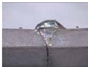
Inadequate joint penetration
