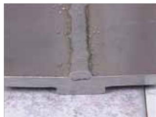
Excessive face reinforcement
