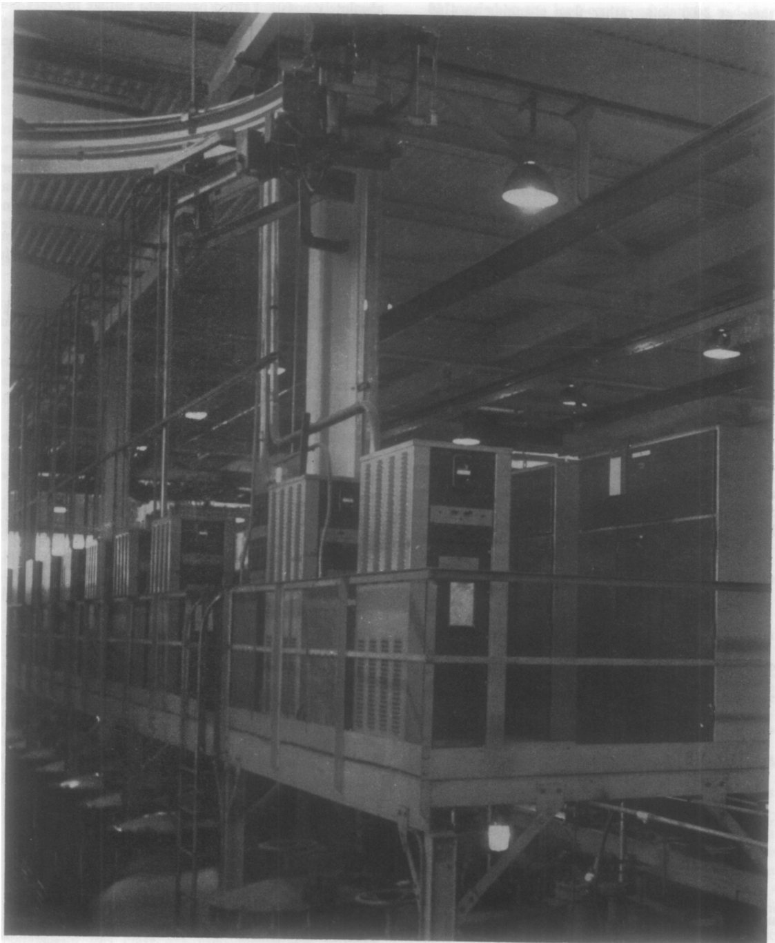
Figure 2.6a A line-up of automatic induction voltage regulators to maintain precise voltage on critical plating lines
