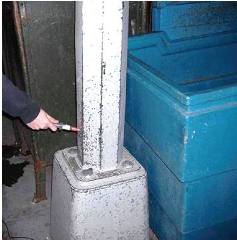
Figure 16—Voltage detection using a pen tester
