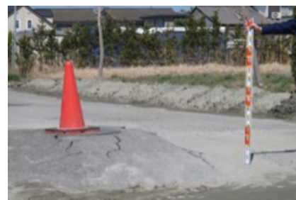
Underground cable duct collapse (Heavy rain)
