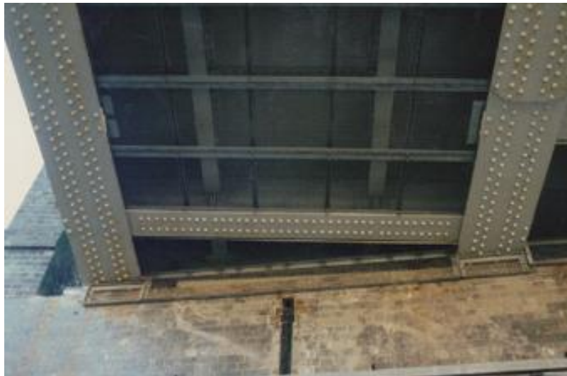
Figure 3 - Structure No. S15 - anti-pigeon mesh prevents access for inspection
