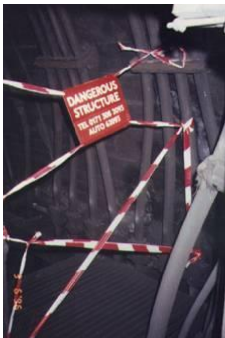
Figure 2 - Structure No. VP84D - Vulnerable Structure notice and hazard tape placed at top of segmental ringed shaft. Notice also placed at base of shaft.
