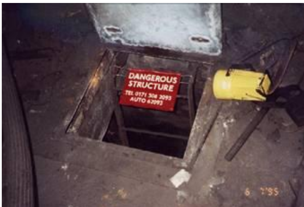
Figure 1 - Structure No. TTR9 - Vulnerable Structure notice attached to loose ladder leading down to platform invert
