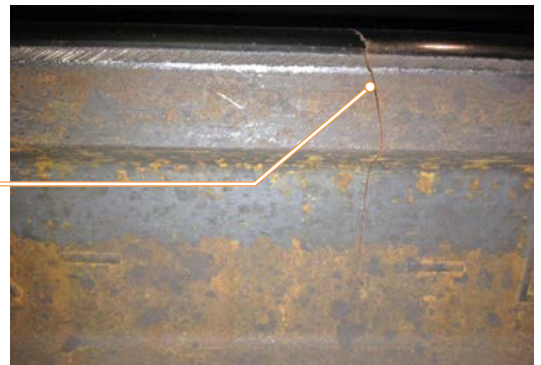
Crack in rail head
