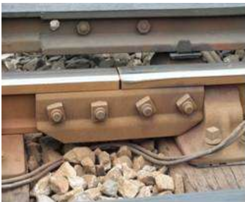
Plate 4 Rail creep: fishplates bearing against a chair
