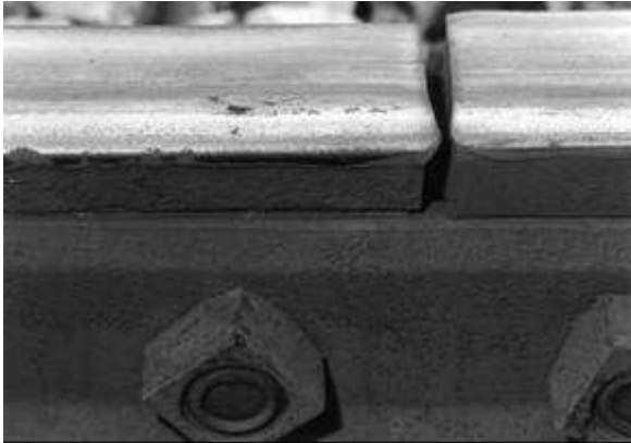
Plate 2 Lipped rail joint
