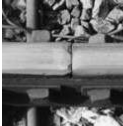
Plate 3 Rail joint with lipping breaking off
