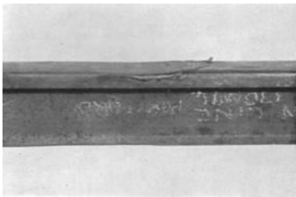
Plate 1 Shallow wheelburn which would benefit from profile grinding. After grinding welding would probably not be required
