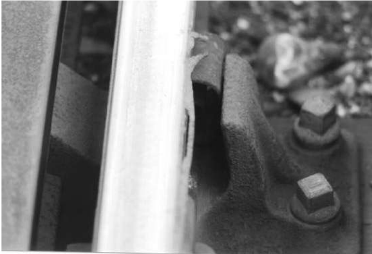
Plate 4 Mushrooming should be removed by grinding otherwise it can lead to cracks developing in the head of the rail. Broken-off strips of steel can also cause signalling short circuits.
