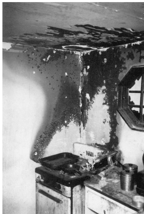
FIGURE 6.11 Clean Burn on Wall Surface.
