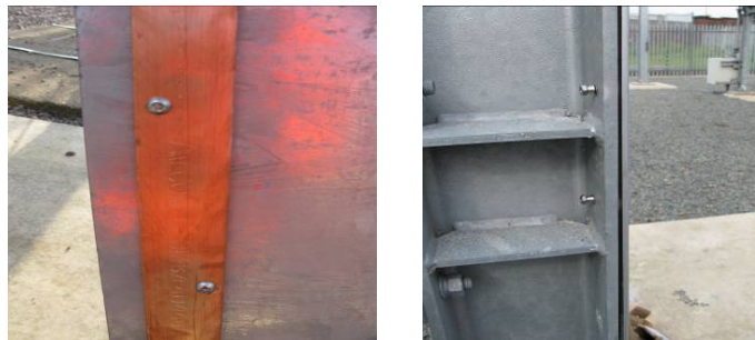
Figure 3 Typical images showing stainless steel keyed bolts and sheer nuts (unsheared)
