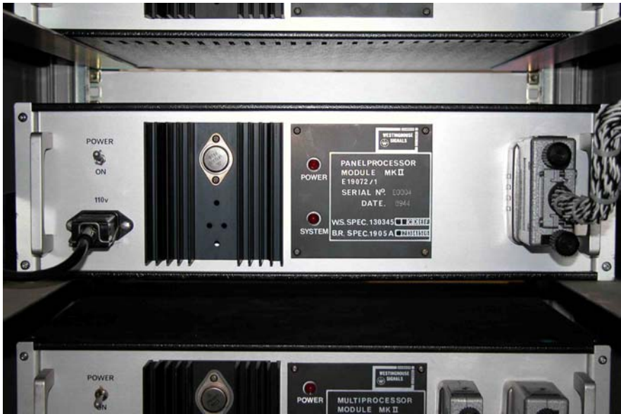
Westinghouse PPM Installed in cubicle
