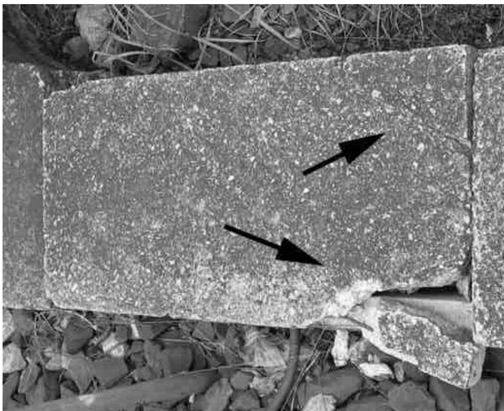
Figure 2 – Exposed reinforcing and damaged corner: replace
