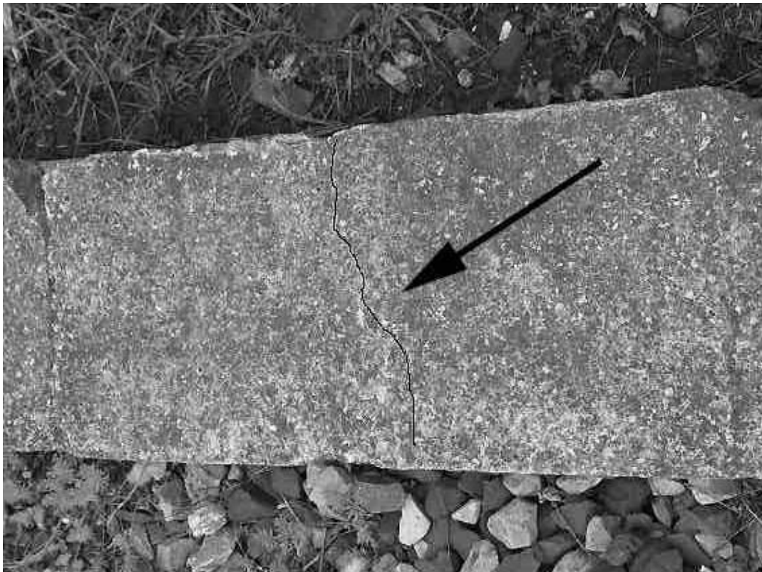
Figure 3 – Unit cracked completely: replace
