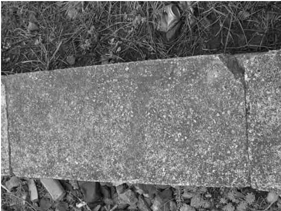
Figure 1 – Damaged corner: replace
