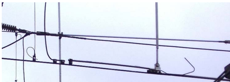
Modified neutral section (with old arcing horn shown)
