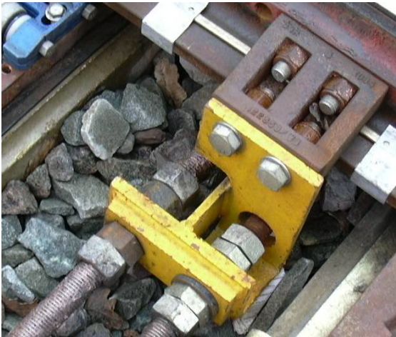
Figure 6 – Installed Corus Cogifer (CC) adjustable stretcher bar assembly (as originally supplied with hard lock nuts)
