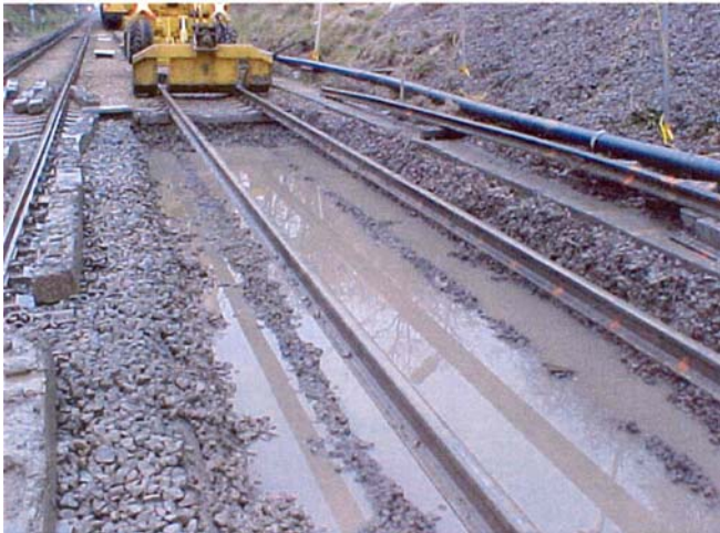
Photo 2: Saturated Track Support System from defective Track Drainage
