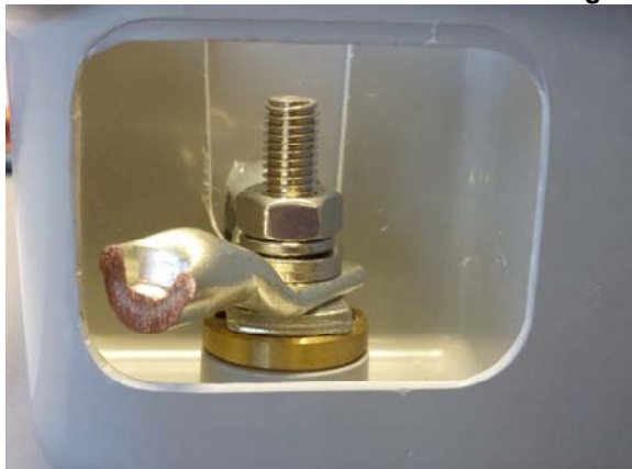
Photo 2: New Build T1/T2 Termination Arrangement
