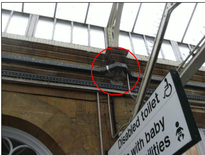
Photograph 1: The original location of the failed section is visible as a pale section in the centre of the picture along with various conduits and cable runs installed over time
