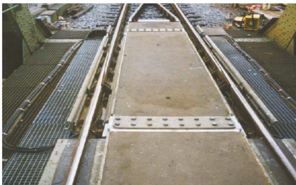
Figure 14 — Rail expansion joint (REJ) in embedded rail
