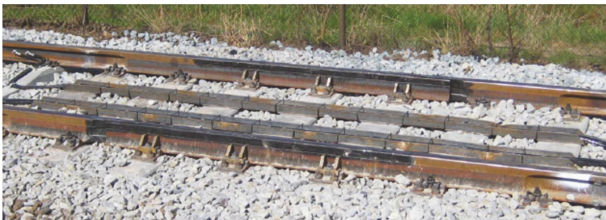
Figure 13 — Rail expansion joint (REJ) in ballasted track
