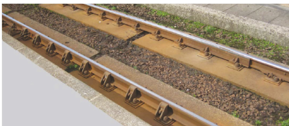
Figure 15 — Rail expansion joint (REJ) in ballastless track
