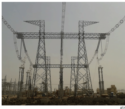
Figure 10 – 1 200 kV single circuit H-type tower (for gantry)
