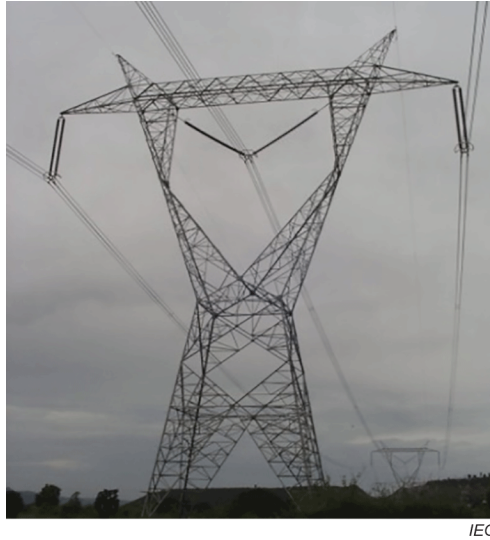
Figure 3 – Typical single circuit horizontal configuration tower
