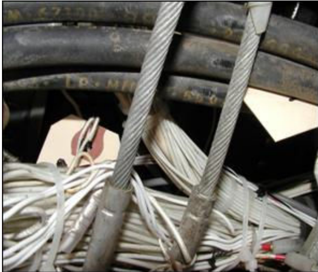
Figure 15 – Example of Inadequate Clearance to Structure
