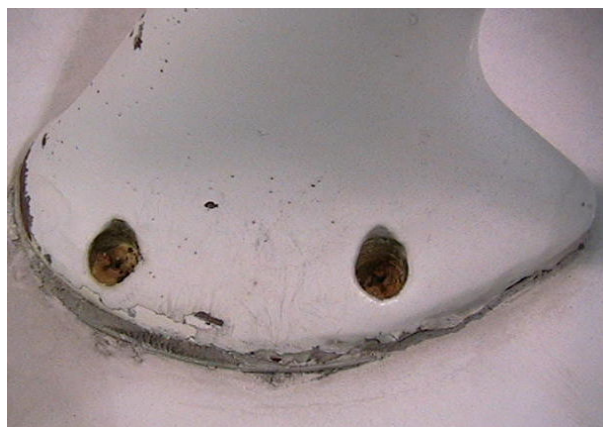
Figure 7 – Corroded Screw Heads
