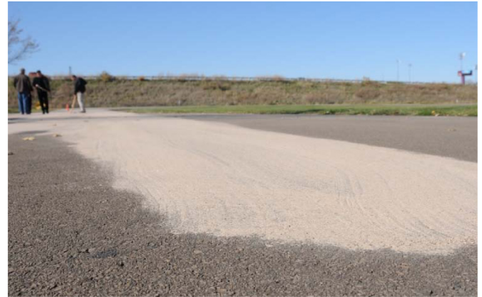
Figure 6. Asphalt Surface with Residual Sand
