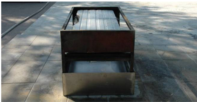
Figure 1. Battery in the support frame placed in a tray
