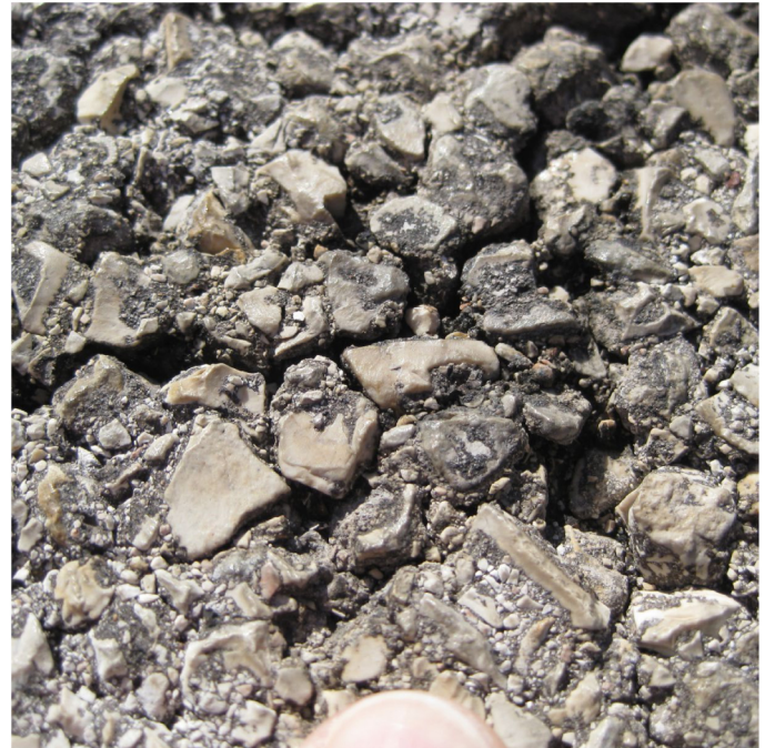
Figure 3. Premature pavement deterioration (raveling) at a joint due to poor construction leading to stripping, where the presence of water causes asphalt binder to separate from the aggregates (rocks and sand).
