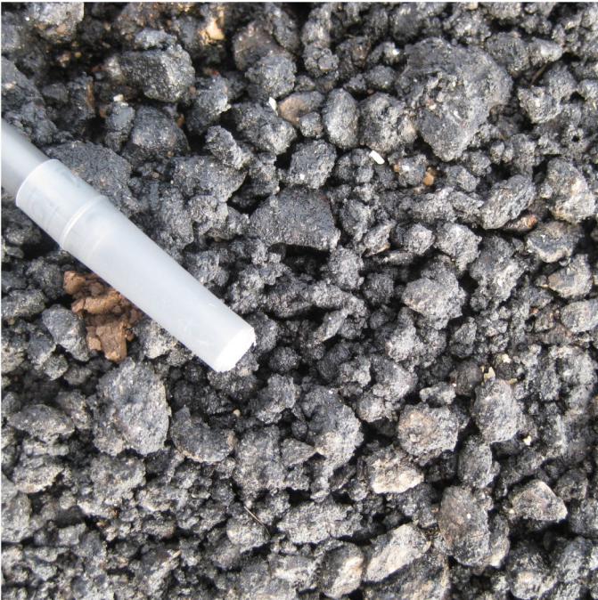
Figure 4. A pavement constructed with a segregated asphalt mixture exhibiting coarse (deep) texture in some areas.
