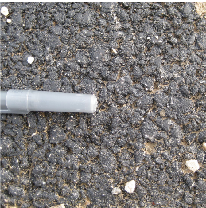
Figure 5. Same pavement in Figure 4 , but at an area approximately 2 m away exhibiting fine (shallow) texture.
