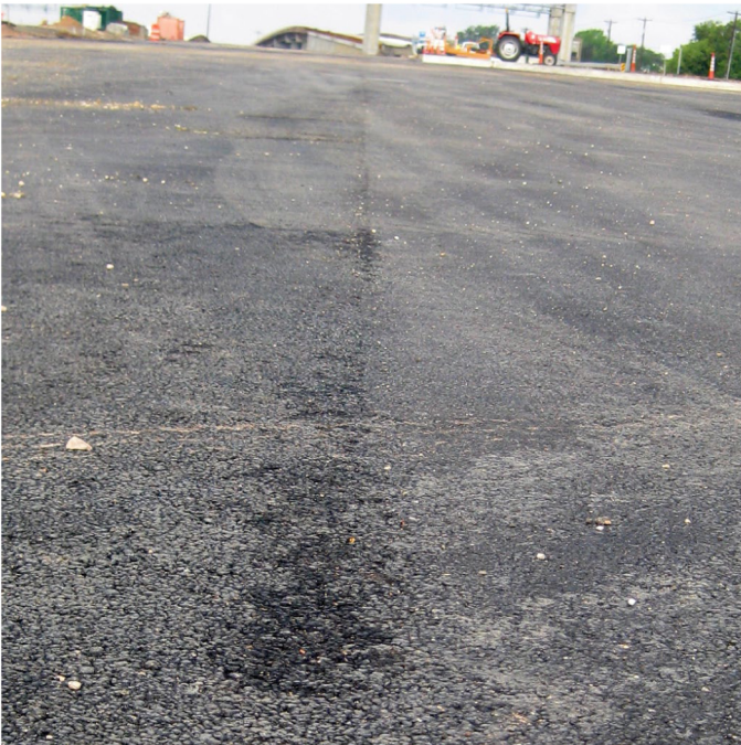
Figure 2. Low joint density allowing for moisture infiltration.
