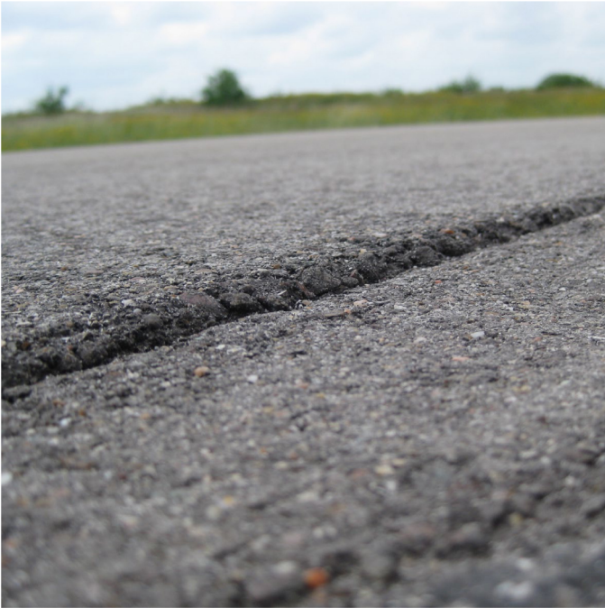
Figure 1. Poor construction can lead to a step across a joint, which can fail compliance with ISO 10844:2011.
