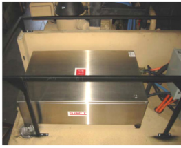
b. SAFT Li-ion battery pack mounted in the truck bed
