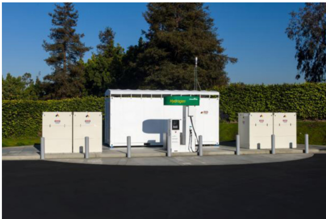
Figure 4. Hydrogen Fueling Station at which MC Default Fill was applied.
