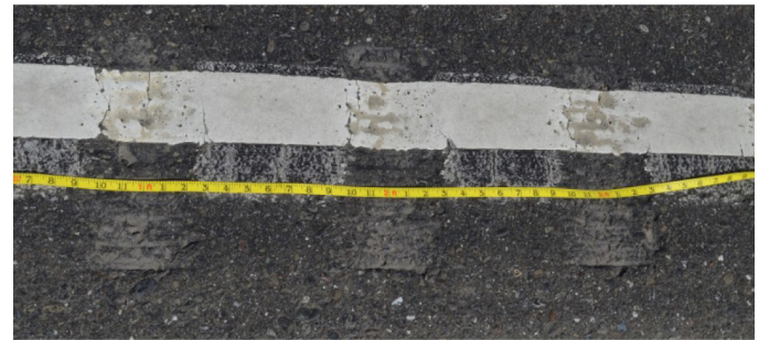
Figure 3. Photograph of the conventional rumble strips found on State Route 299
