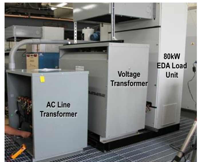
Figure 4. One module of the load emulators used by the EPS showing the load emulator and associated transformers.
