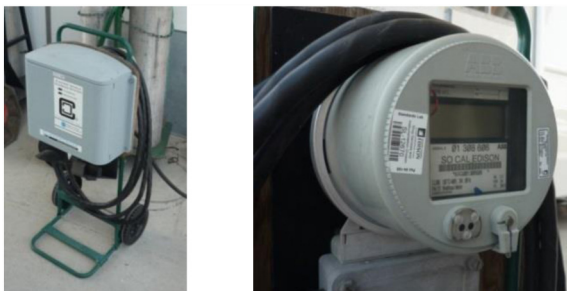
Figure 5. Portable EVSE used for recharging the vehicle
