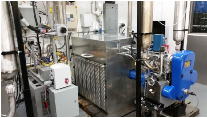
Figure 1. Single cylinder engine (right) and boost/EGR control system (left) as installed in the test cell.
