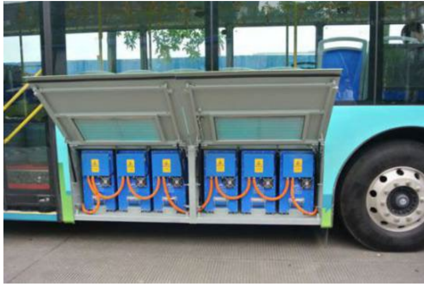
Figure 4 - Battery packs located in the cargo bay Source: Alibaba
