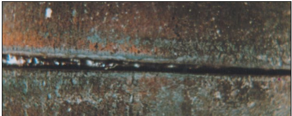
Figure 2.12—Incomplete Joint Penetration
