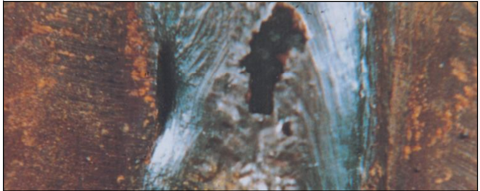
Figure 2.7—Incomplete Fusion at the Groove Face
