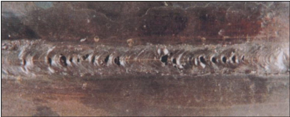
Figure 2.22—Longitudinal Crack and Linear Porosity
